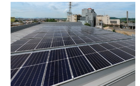
Using renewable energies for in-house generation (Hayashibara Co., Ltd.)
