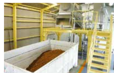
Sludge Reduction Equipment
